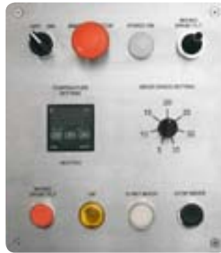
76-PV0077/B Detail of control panel
